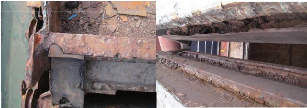
4-2 Seriously corroded rubber channel and draining channel
