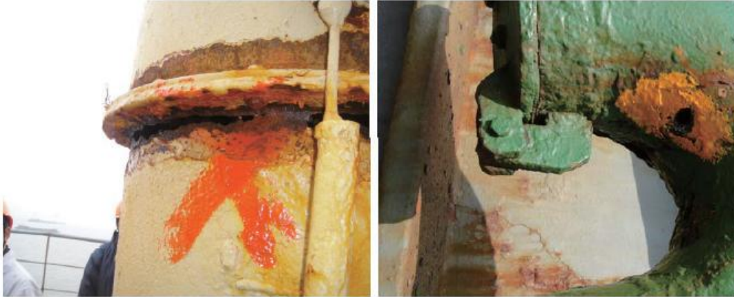
Figure 6 Holed ventilator and air pipe
