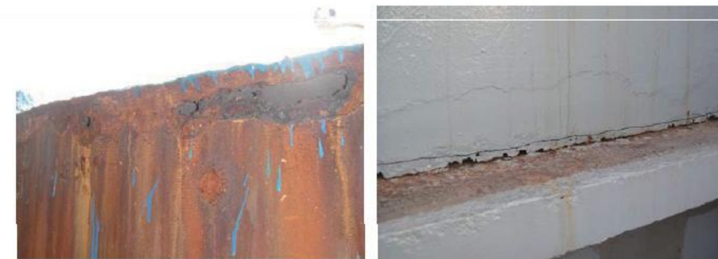
4-3 Seriously corroded skirt plate
